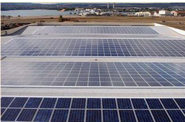
Solar electric panels on rooftop at U.S. Naval Station Pearl Harbor generate enough power for 300 homes.
